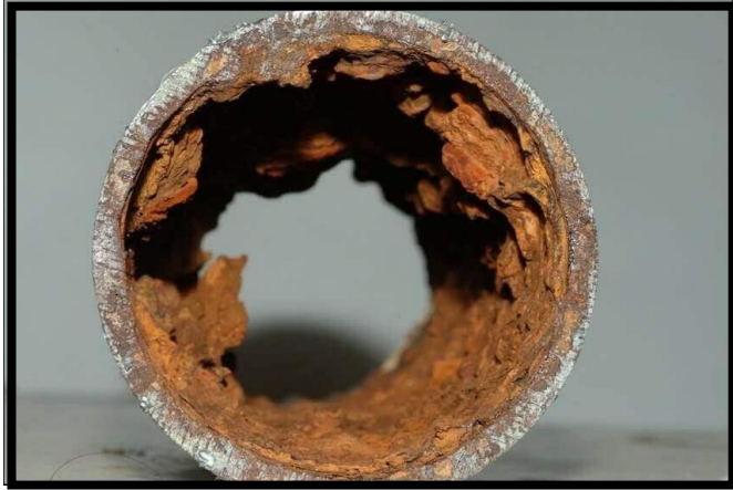
Fig. 1: Corrosion within drinking water pipe
